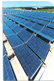
Solar Power Generation Systems
